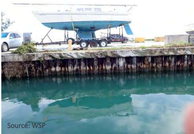
Photo 46: GDP Marina (Deteriorated Sheet Pile Wall)
