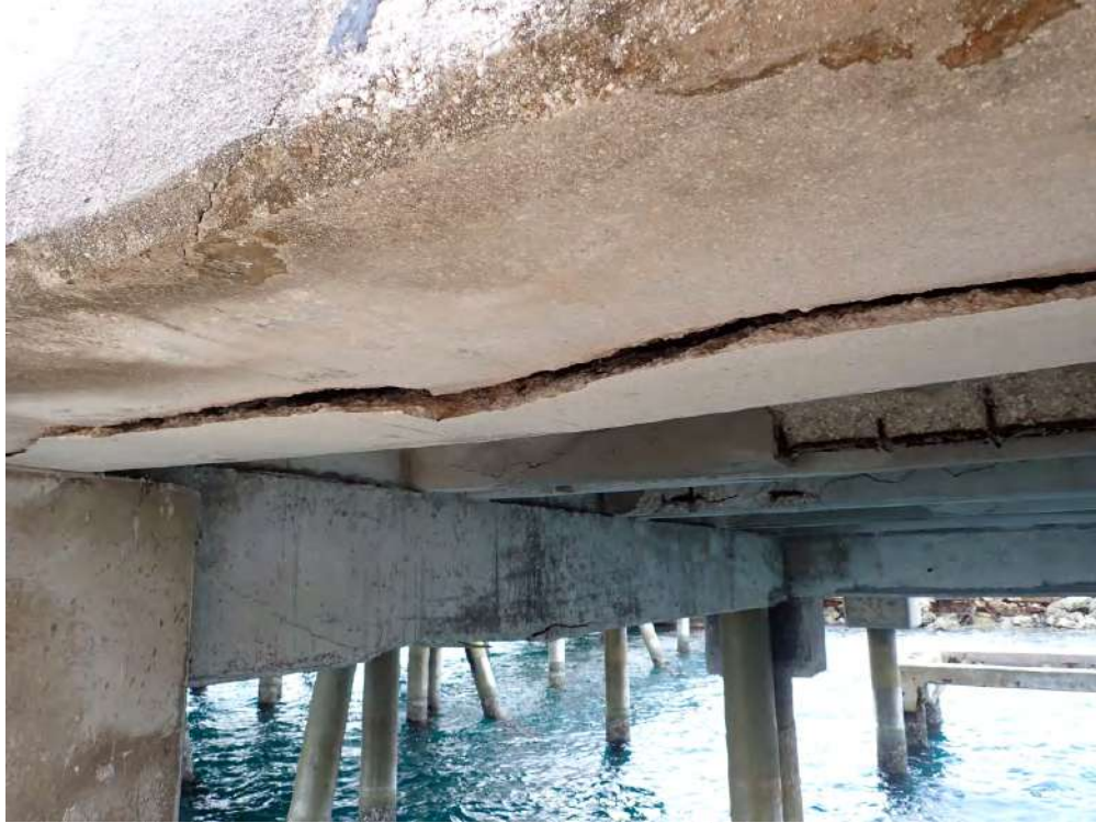
Photo 3 – Crack at Waterside Pile Cap
