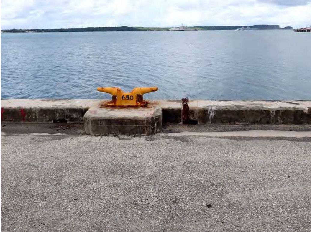
Photo 7 – Berth F3 Typical Corrosion at Mooring Hardware
