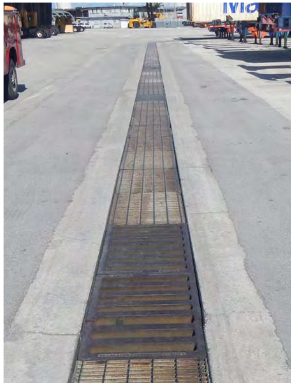
Photo 24: Container Yard Trench Drains
