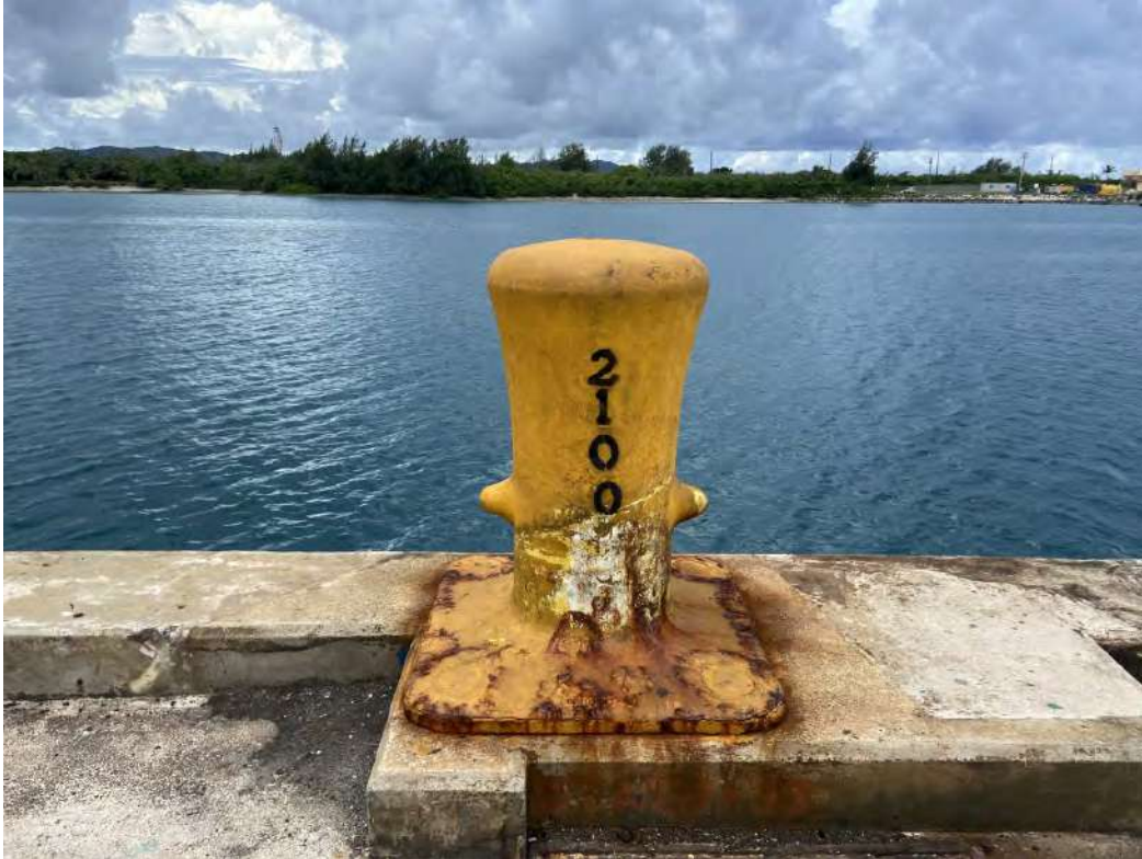
Photo 21 – Berth F6 Typical Corrosion at Mooring Hardware
