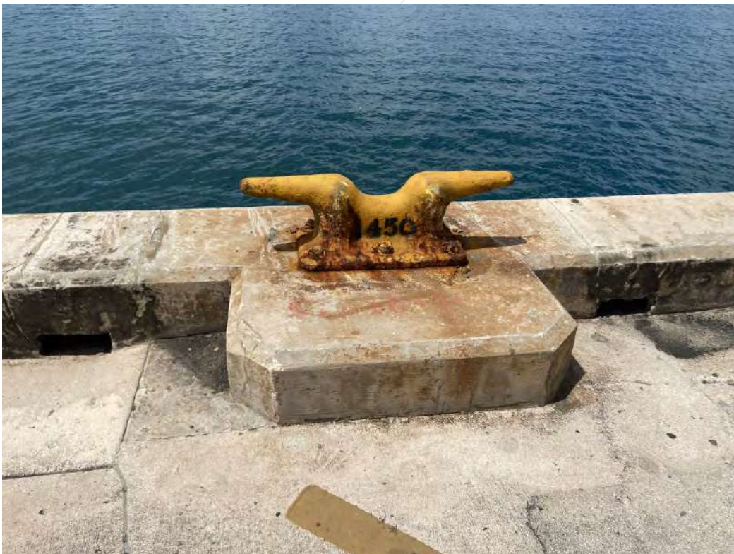
Photo 14 – Berth F5 Typical Corrosion at Mooring Hardware
