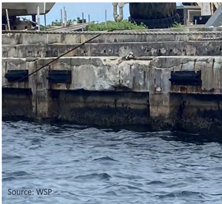
Photo 34: Hotel Wharf (Open-Corrosion Spalling)
