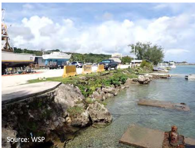
Photo 47: GDP Marina (Erosion on North Side of Breakwater)
