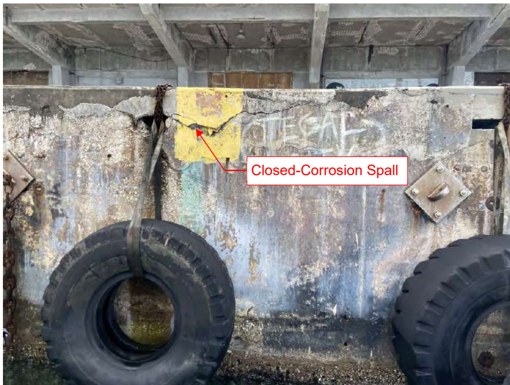
Photo 6 – Berth F3 Typical Closed-Corrosion Spalling
