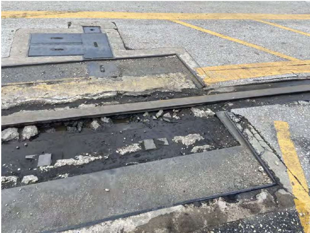
Photo 16 – Berth F5 Damage at Asphalt Overlay
