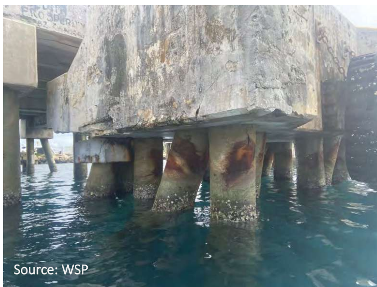
Photo 26: Breasting Dolphin H (Failed Repair and Damaged Fender System)
