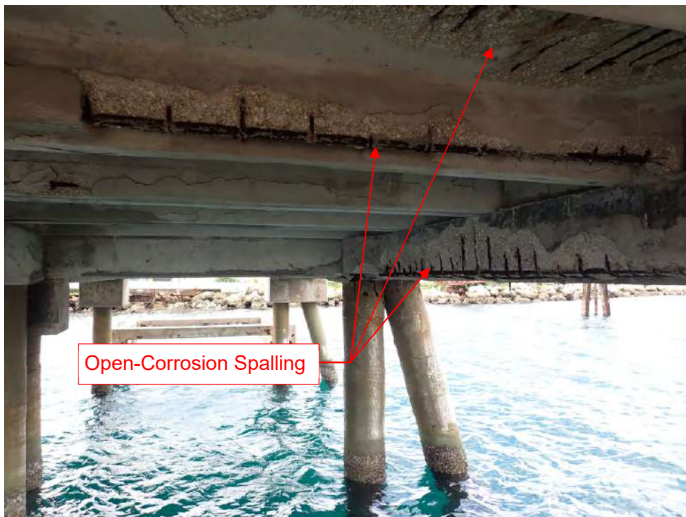
Photo 2 – Open Corrosion Spalling
