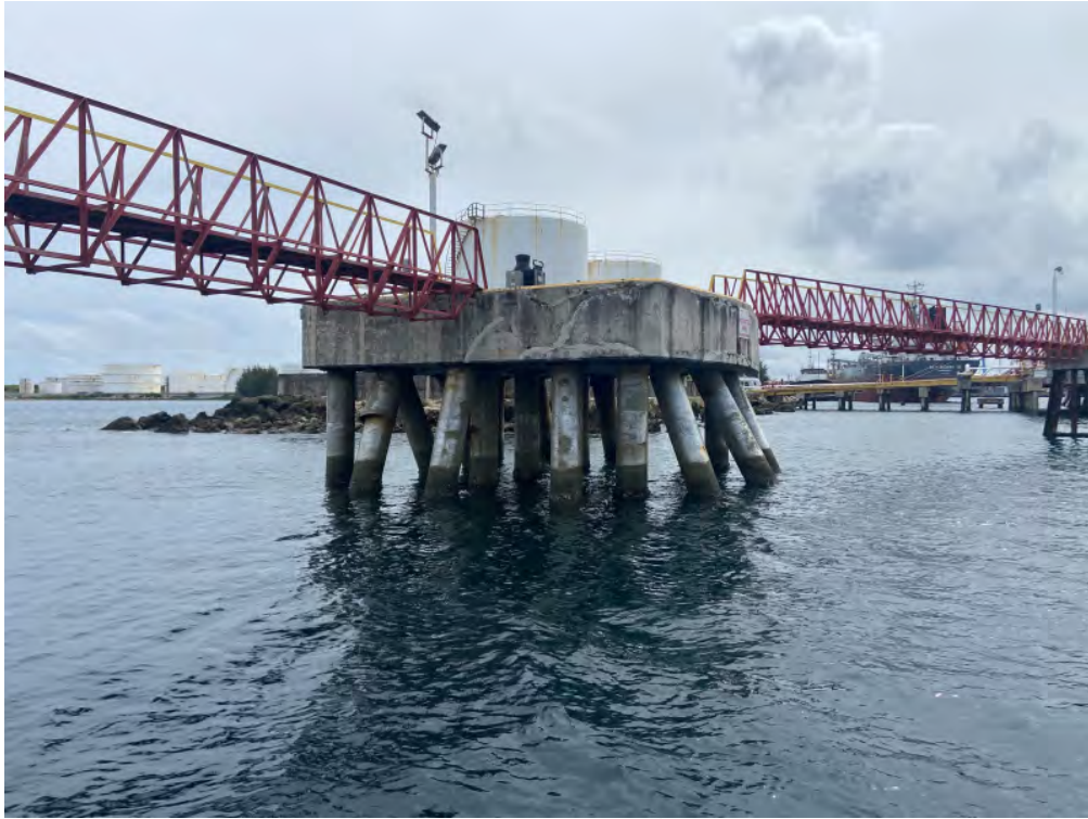
Photo 9 – Mooring Dolphin B
