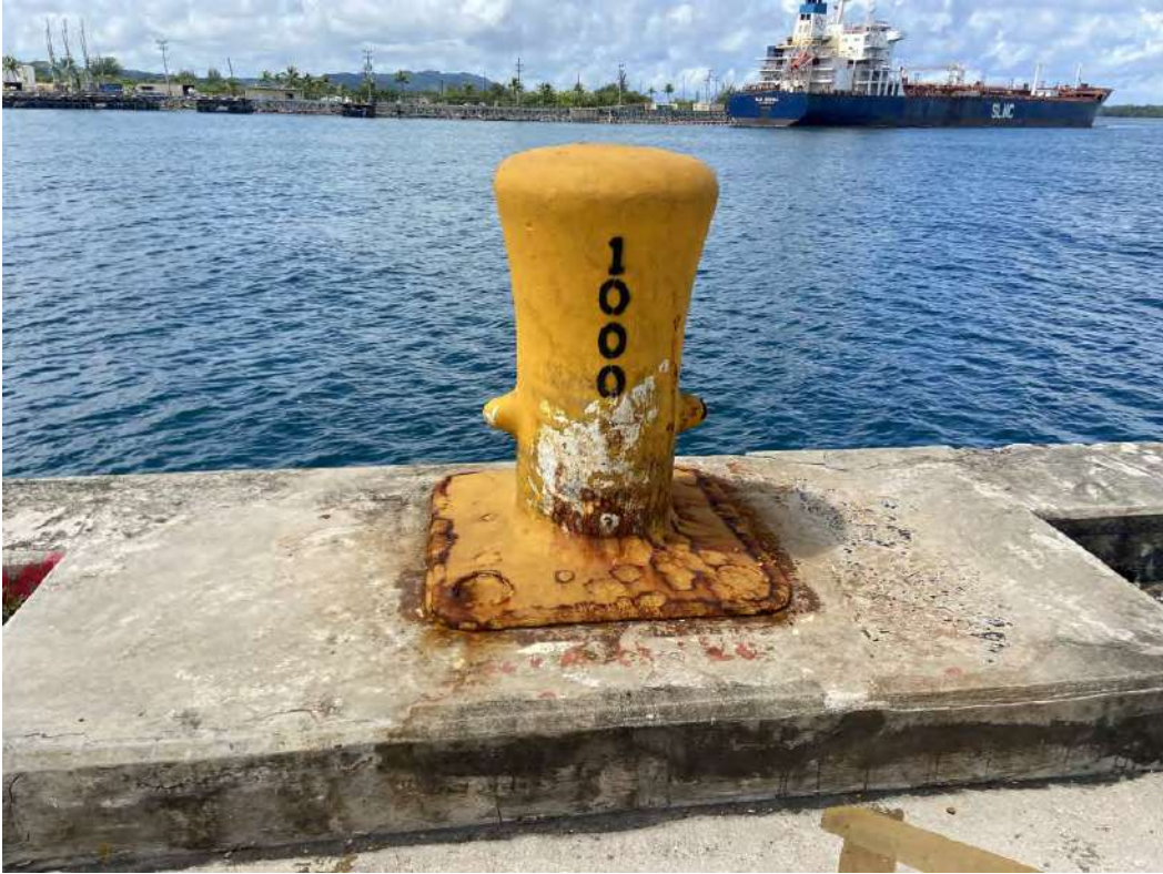
Photo 9 – Berth F4 Typical Corrosion at Mooring Hardware
