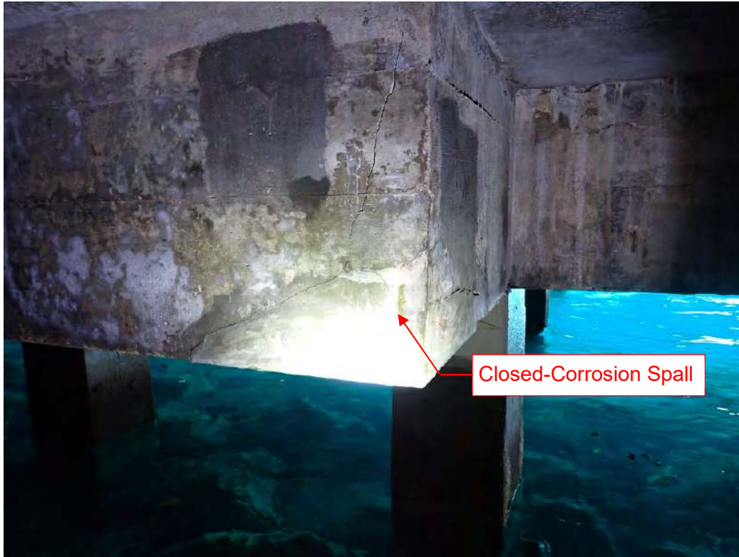
Photo 19 – Berth F5 Closed Corrosion Spall at Pile Cap
