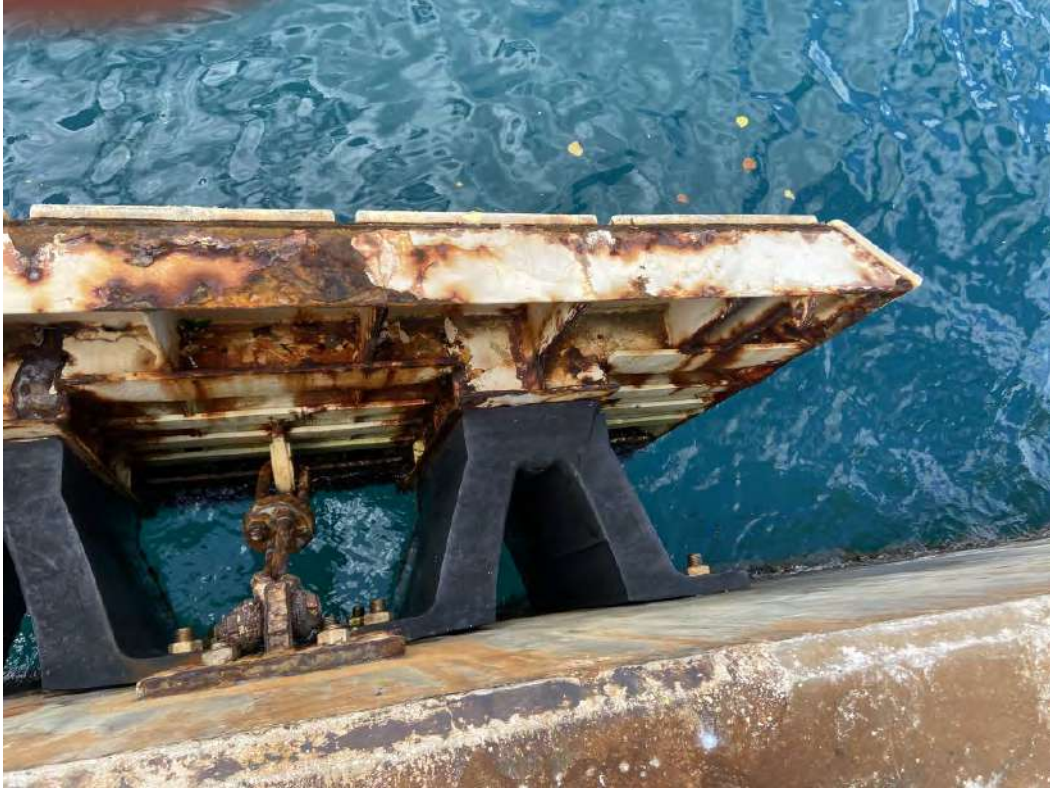
Photo 15 – Typical Fender Panel
