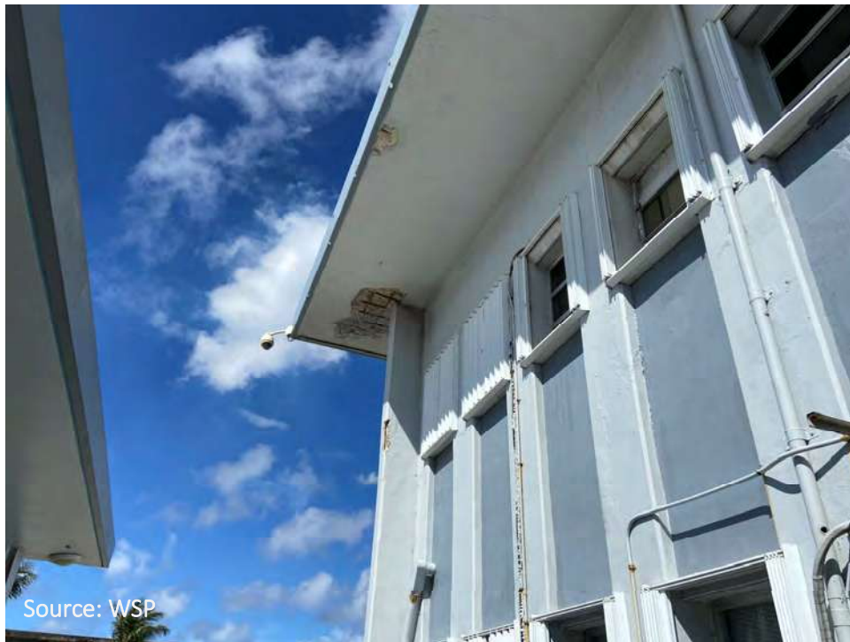
Photo 10: Administration Building Concrete Spalling
