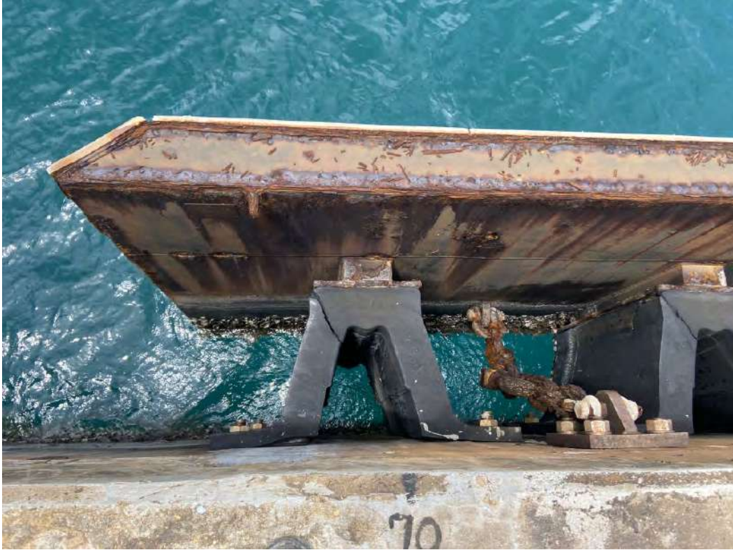
Photo 17 – Berth F5 Typical Damaged Fender Elements
