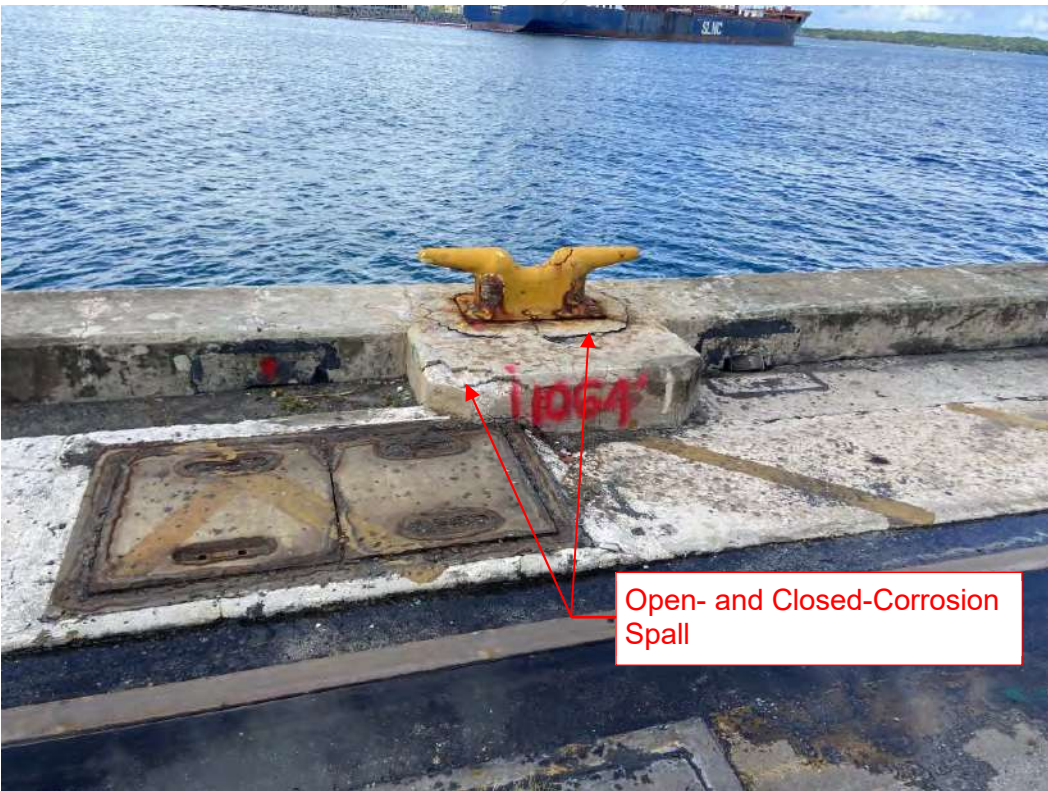
Photo 10 – Berth F4 Concrete Spall at Bullrail/Cavel
