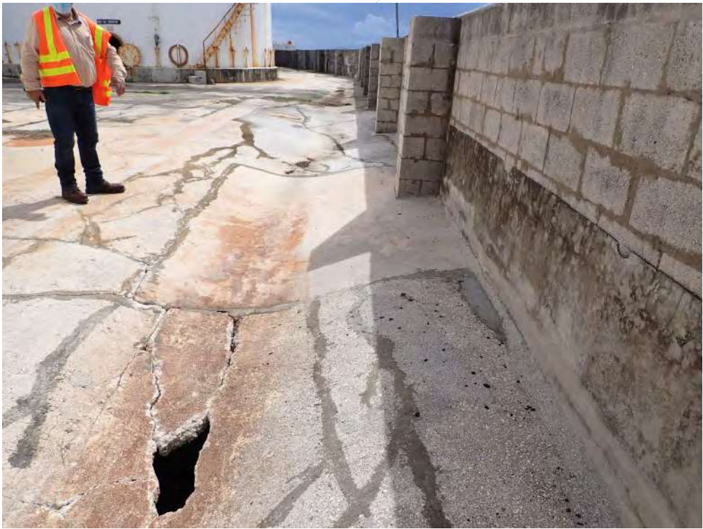
Photo 6 – Void and Settlement at North Side of Peninsula
