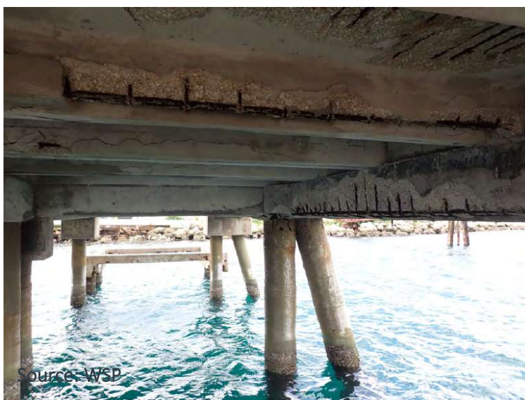
Photo 25: Main Pier (Open Corrosion Spalling)
