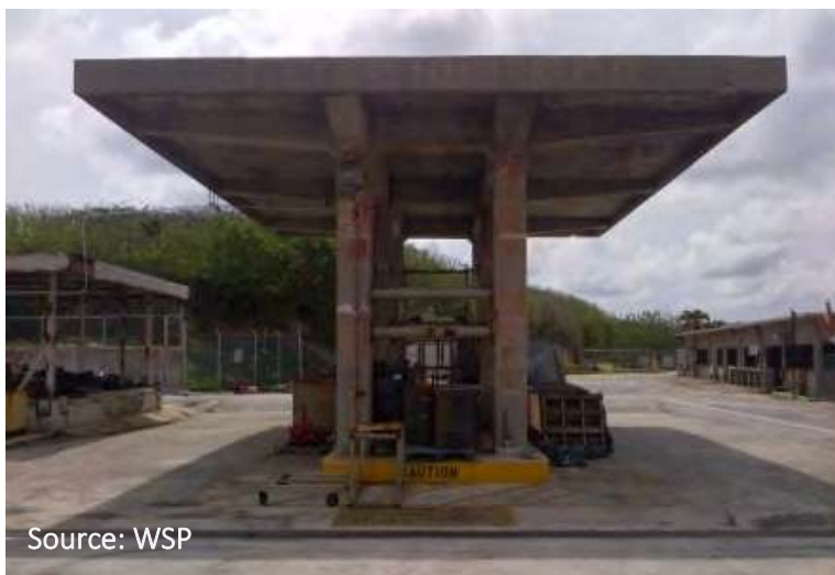
Photo 36: Truck Loading Facility
