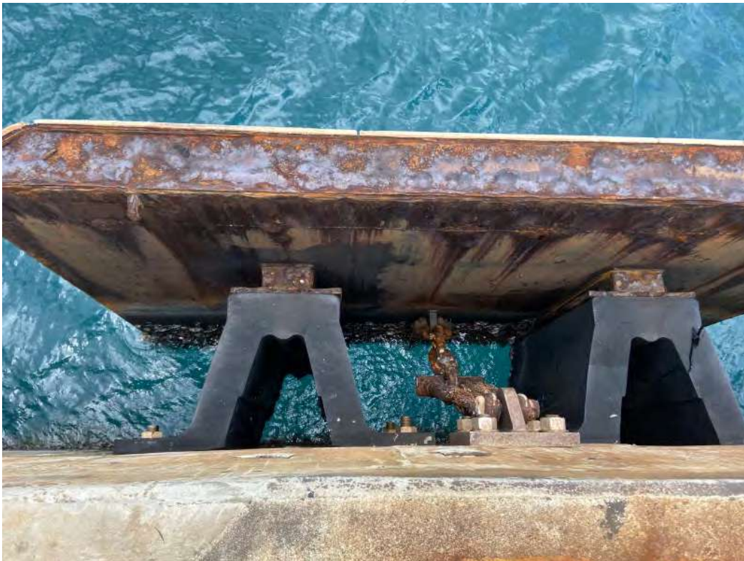
Photo 22 – Typical Fender Panel
