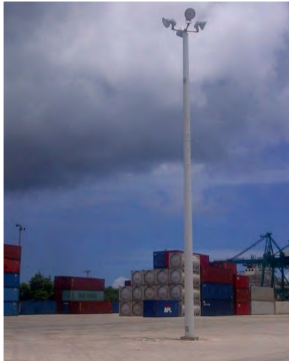
Photo 23: Container Yard Light Pole
