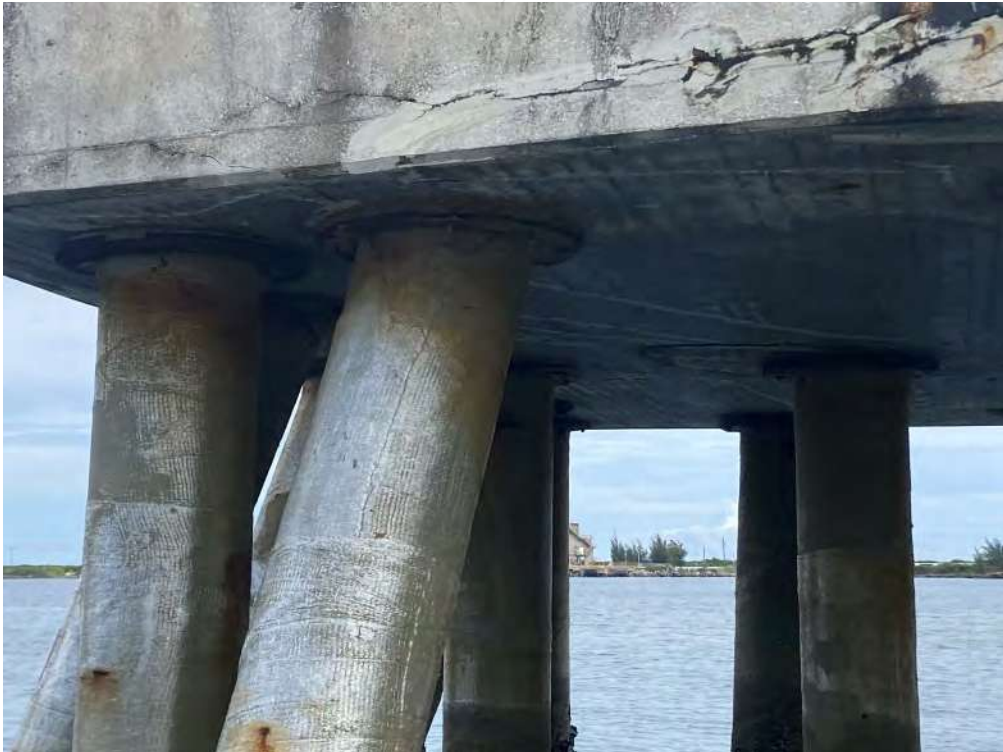
Photo 10 – Mooring Dolphin B
