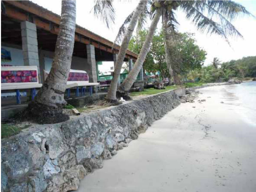
Figure 77. Grouted CRM wall protecting Agat Mayor’s Office in the foreground. Teal pavilions in the background are part of Agat Sagan Bisita.
