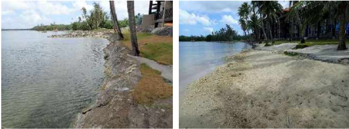
Figure 71. Inn on the Bay property, looking north. Typical of northern section on the left, with no beach fronting the wall. Typical southern section on the right, where a sandy beach starts to form.
