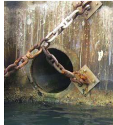
Figure 4: Untreated Storm Water Flowing Directly into Apra Harbor
