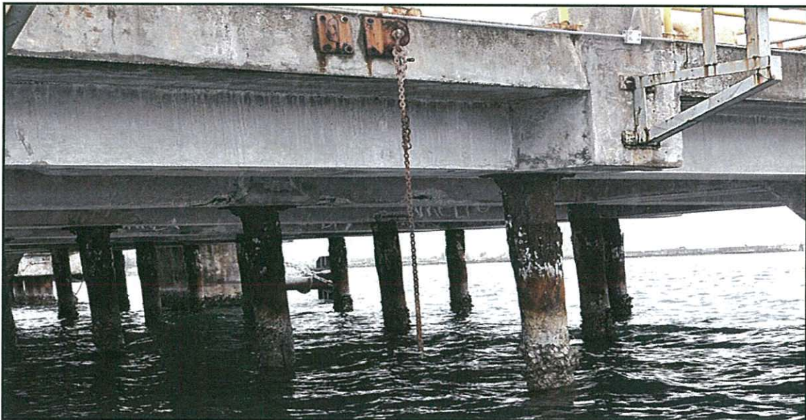
Golf Pier Boat Tour: The pier beams and steel piles at Golf Pier was one of the sites toured with the Port and WSP team members. In addition the group also toured F-1 and H-Wharf.
