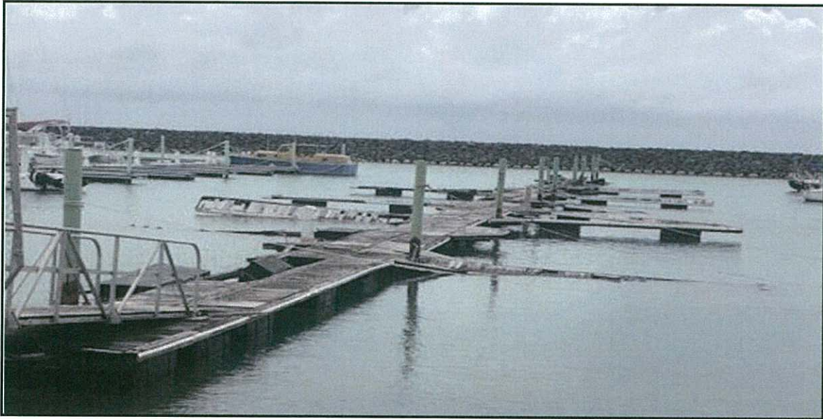
Agat Marina, most of Dock B remained intact, but sustained further damage by the typhoon. A contractor, Canton Construction, has already been obtained by the Port to demolish Dock B.
