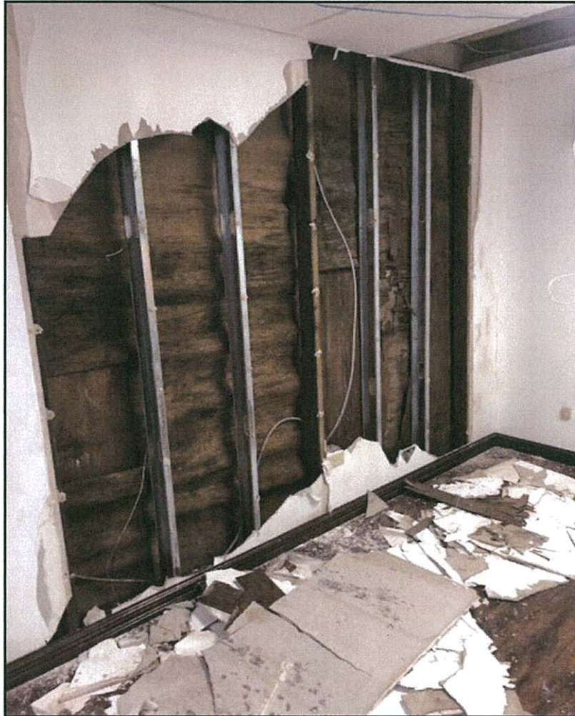
Mold found at the Safety Office building.
