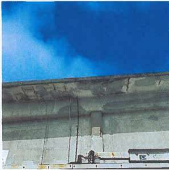
Figure 6: Concrete Spalls to be Repaired (East Overhang)
