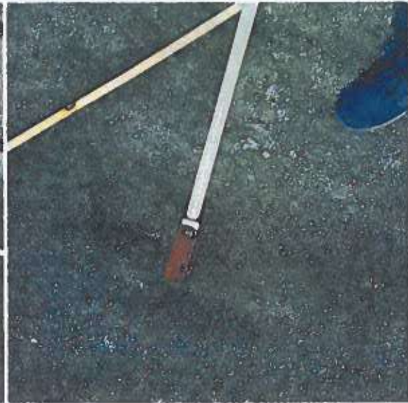
Figure 13: Electrical Line to be Removed and Relocated
