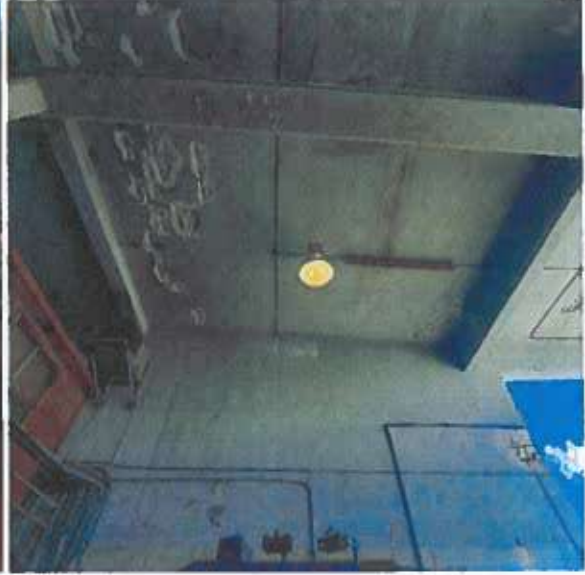
Figure 20: Light Fixture and Conduit to be Replaced
