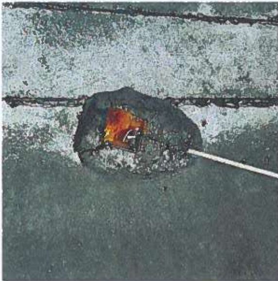
Figure 12: Electrical line to be Removed and Relocated
