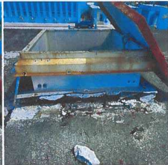
Figure 15: Concrete Collar to be Repaired
