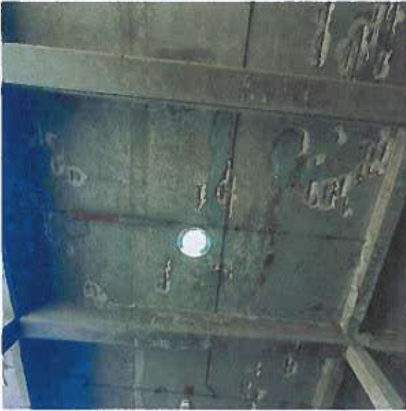
Figure 8: Concrete Spalls to be Repaired (Interior Ceiling)
