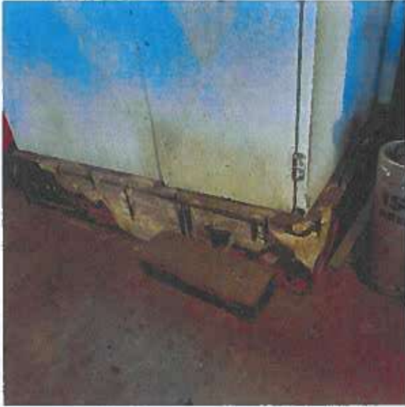
Figure 19: Bathroom Foundation to be Repaired
