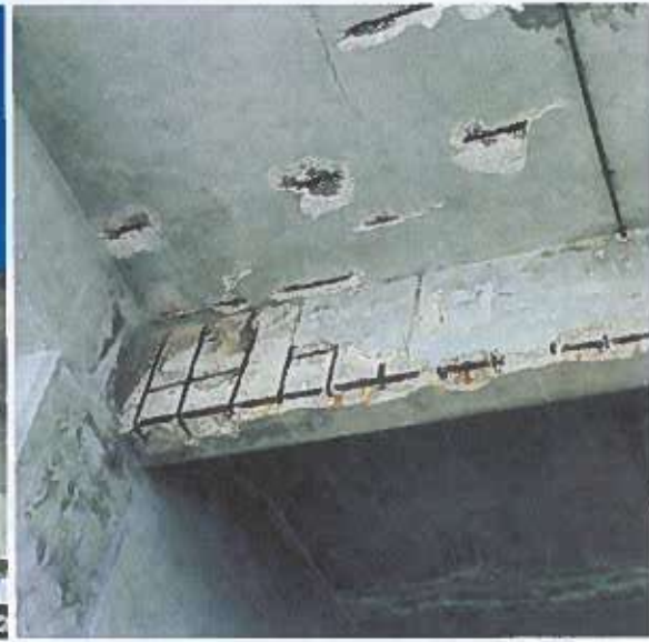
Figure 7: Concrete Spalls to be Repaired (South Elevation)
