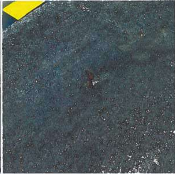
Figure 9: Fall Protection Anchor to be removed (Rooftop)
