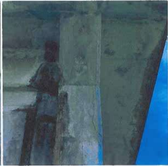
Figure 5: Concrete Spalls to be Repaired (North Elevation)
