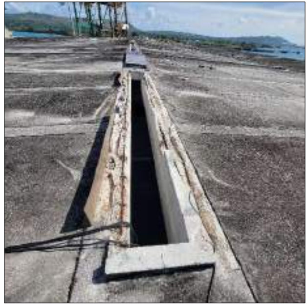
Figure 26: Bay 12 – Concrete curb to be repaired/rebuilt.
