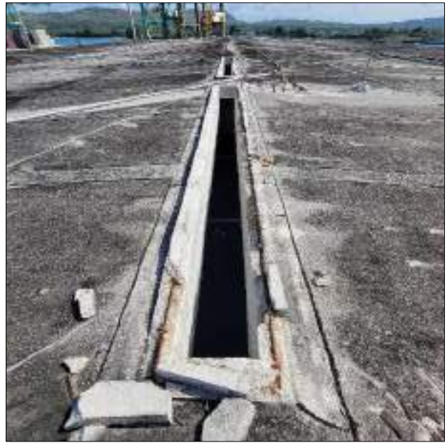
Figure 22: Bay 10 – Concrete curb to be repaired/rebuilt.
