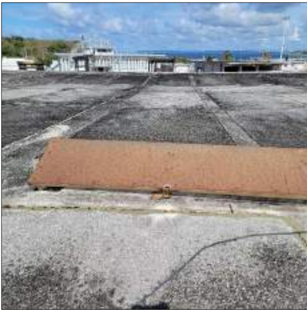
Figure 15: Bay 7 – Welds have failed and the roof vent is no longer connected to the concrete curb.
