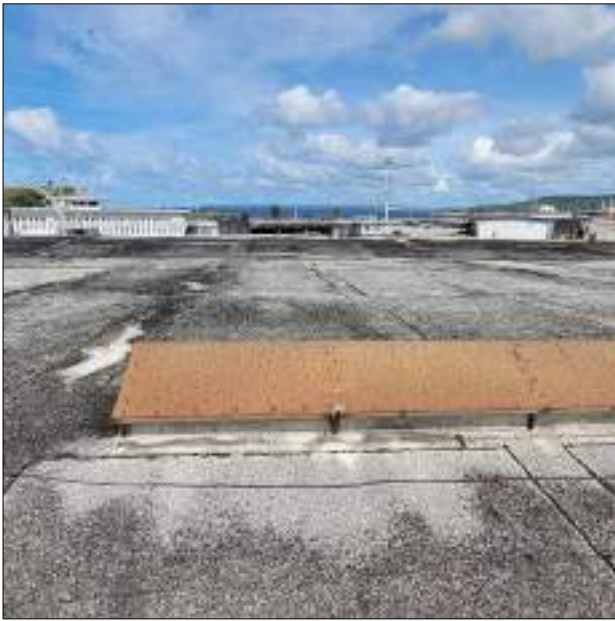
Figure 9: Bay 5 – Welds have failed and the vent has shifted.
