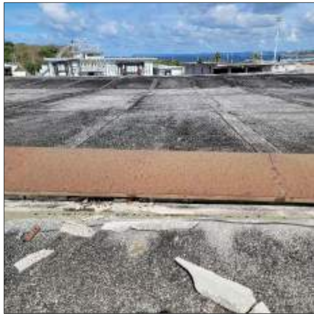
Figure 16: Bay 7 – Concrete curb to be repaired/rebuilt.
