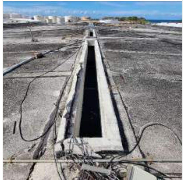
Figure 20: Bay 9 – Concrete curb to be repaired/rebuilt.
