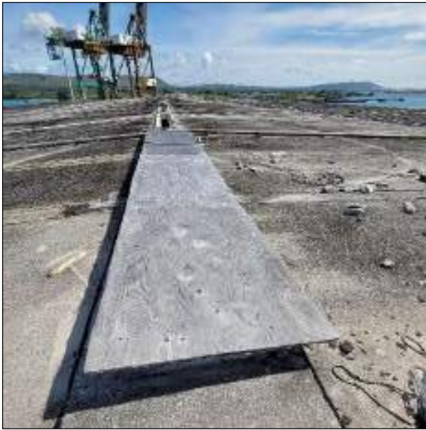
Figure 25: Bay 11 – Concrete curb to be repaired/rebuilt.
