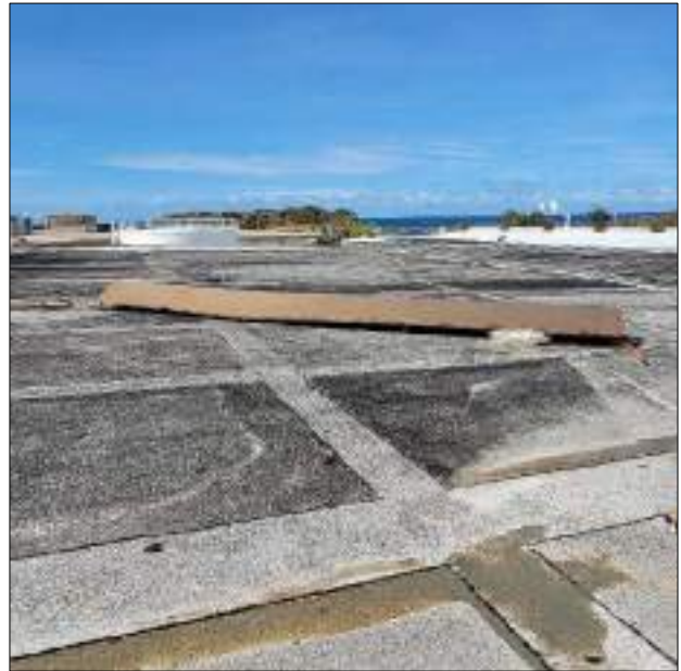
Figure 36: Near Bay 12 & 13 – Roof vent to be disposed.
