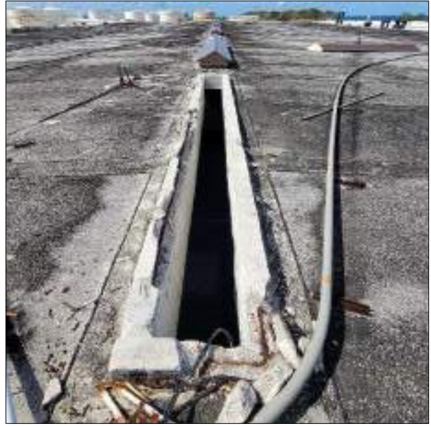
Figure 2: Bay 2 – Roof vent opening. Concrete curb to be repaired/rebuilt.
