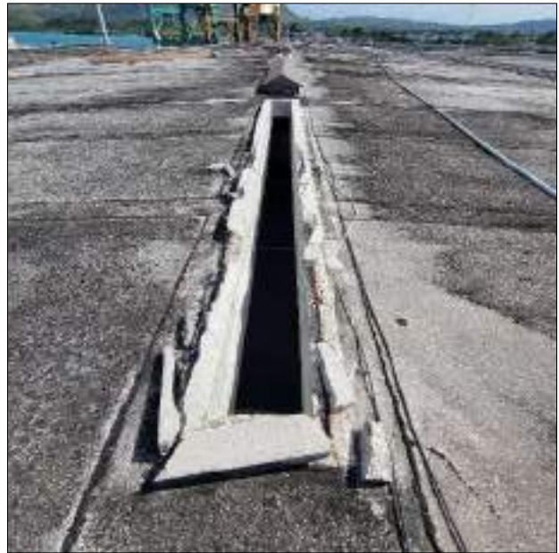
Figure 12: Bay 6 – Concrete curb to be repair / rebuilt.
