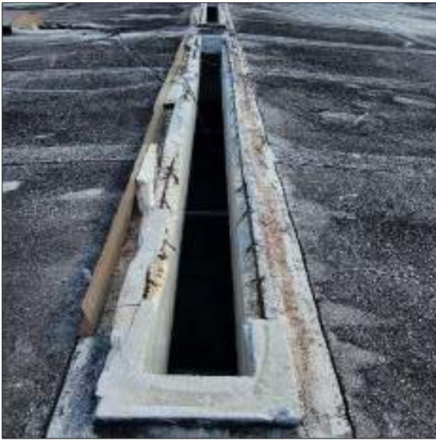
Figure 29: Bay 13 – Concrete curb to be repaired/rebuilt.
