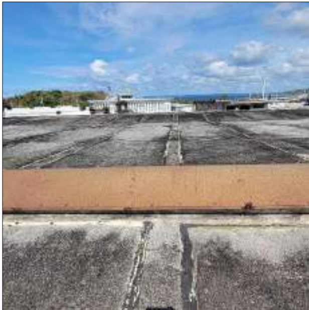
Figure 19: Bay 8 – Concrete curb to be repaired/rebuilt.
