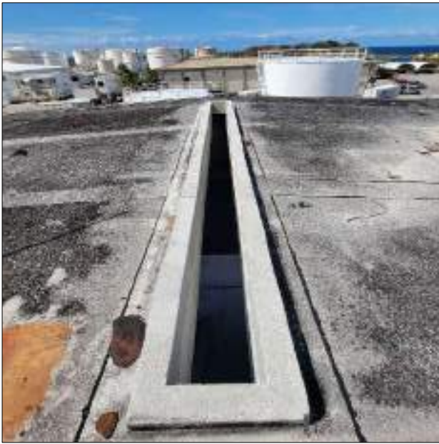
Figure 33: Bay 15 – Concrete curb to be repaired/rebuilt.
