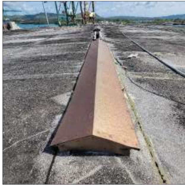
Figure 14: Bay 7 – Roof vent to be disposed.
