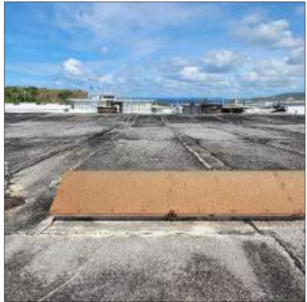
Figure 18: Bay 8 – Welds have failed and the vent is no longer connected to the concrete curb.
