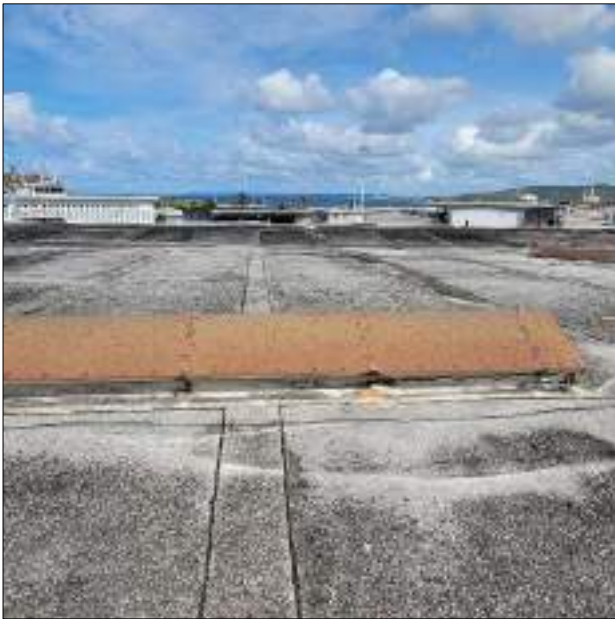
Figure 11: Bay 5 – Concrete curb to be repaired.
