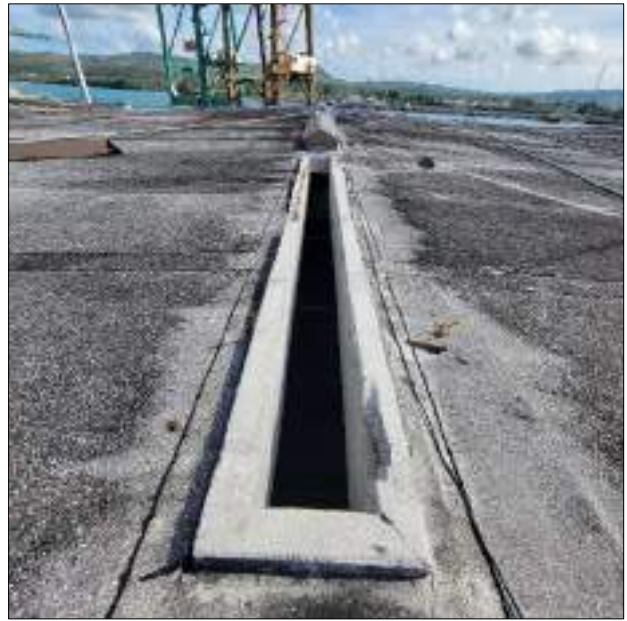
Figure 6: Bay 4 – Roof vent opening. Concrete curb to be repaired /rebuilt.
