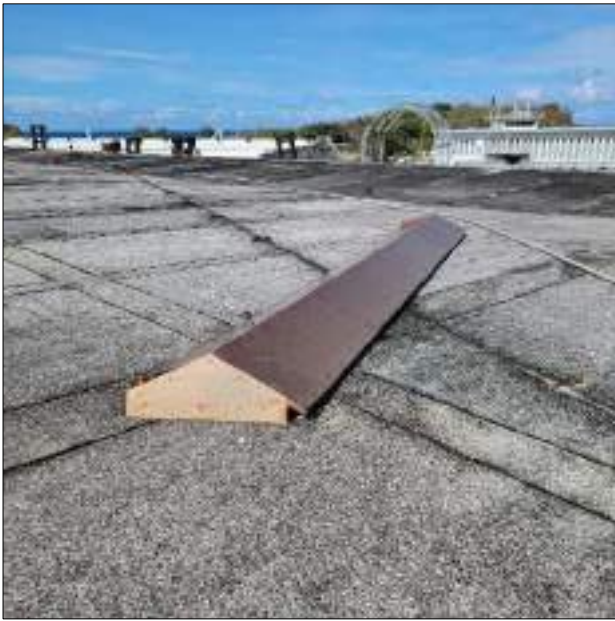
Figure 37: Near Bay 3 & 4 – Roof vent to be disposed.
