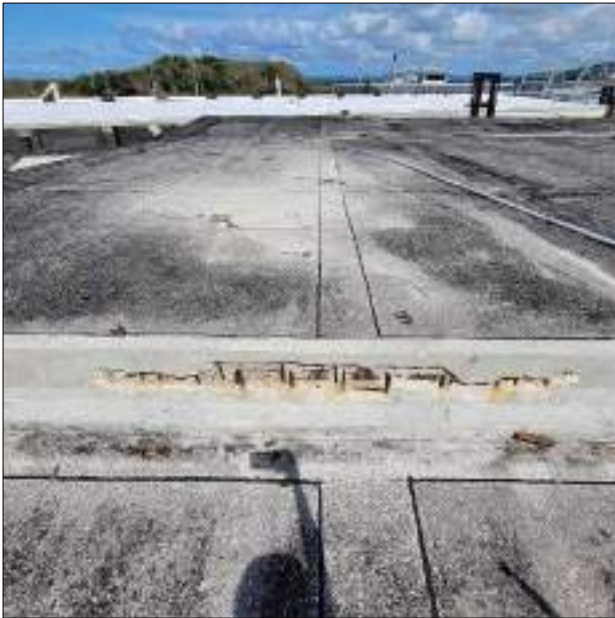
Figure 35: Bay 15 – Concrete curb to be repaired. Concrete curb has a height of 31" from top to bottom.
