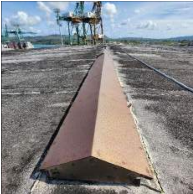
Figure 17: Bay 8 – Roof vent to be disposed.
