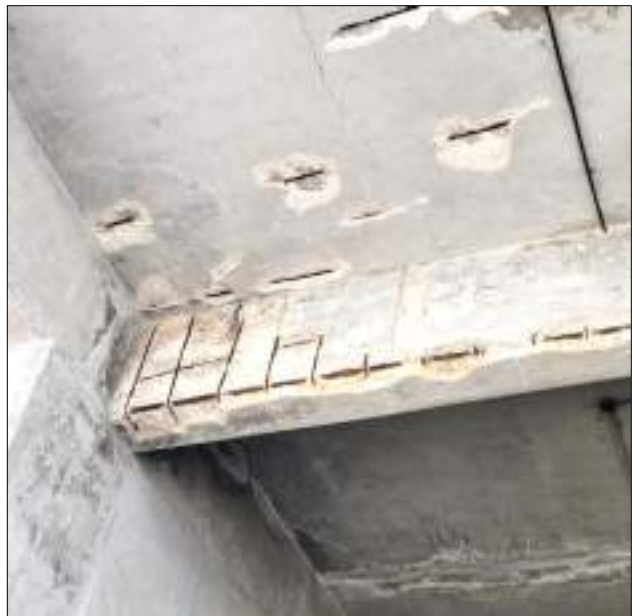
Figure 7: Concrete Spalls to be Repaired (South Elevation)
