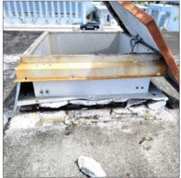
Figure 15: Concrete Collar to be Repaired
