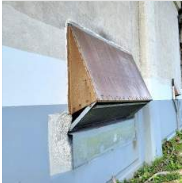
Figure 3: Exhaust Vent to be Removed and Replaced
