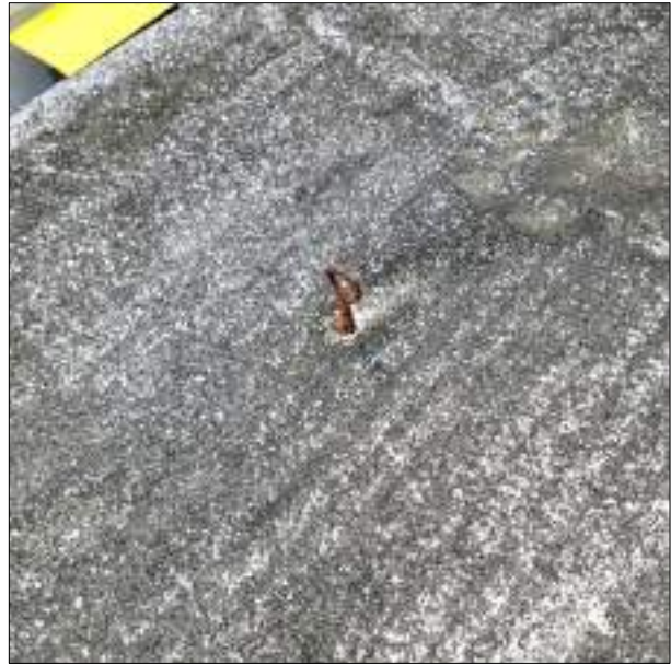
Figure 9: Fall Protection Anchor to be removed (Rooftop)
