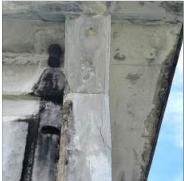
Figure 5: Concrete Spalls to be Repaired (North Elevation)
