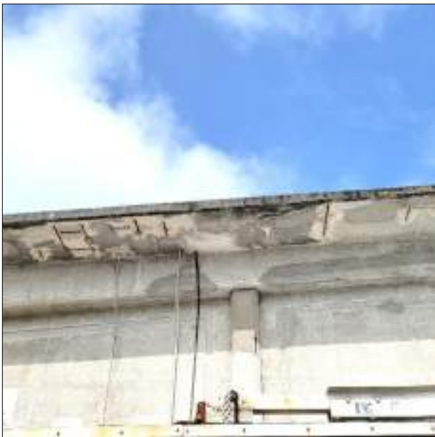
Figure 6: Concrete Spalls to be Repaired (East Overhang)
