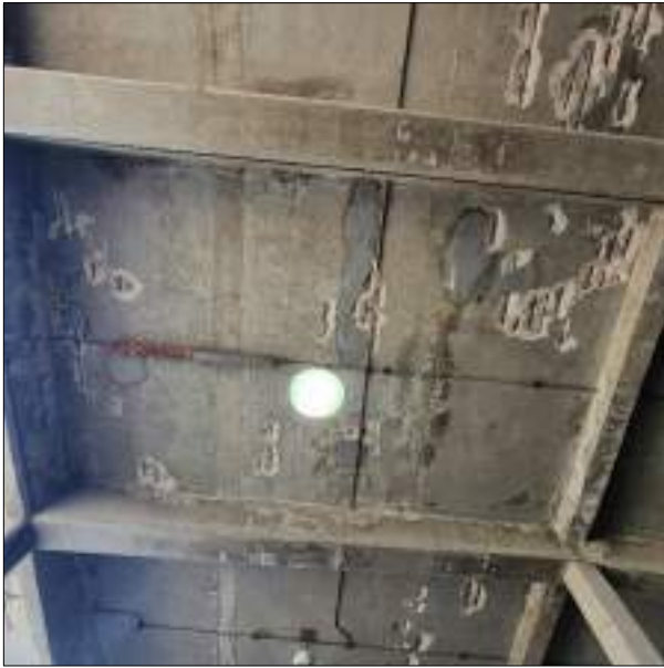
Figure 8: Concrete Spalls to be Repaired (Interior Ceiling)
