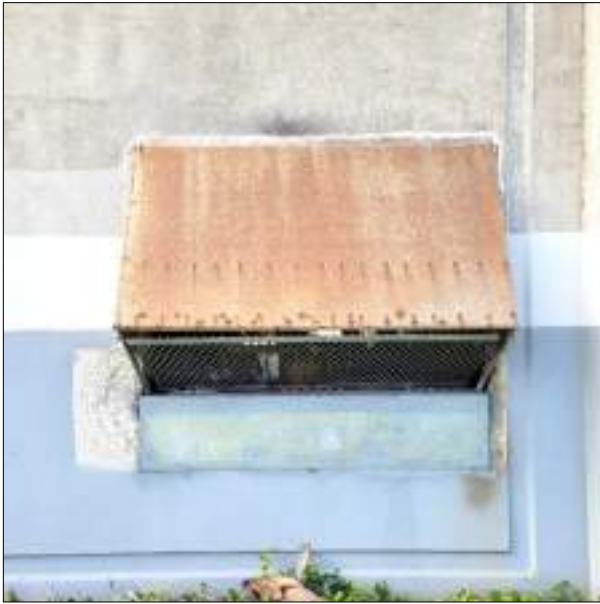
Figure 1: Exhaust Vent to be Removed and Replaced
