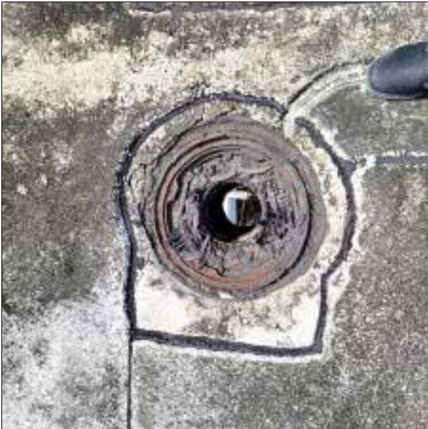
Figure 10: Roof Drain to be Removed and Replaced
