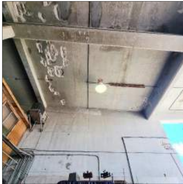
Figure 20: Light Fixture and Conduit to be Replaced
