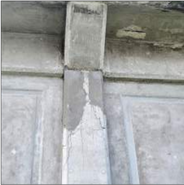
Figure 4: Concrete Spalls to be Repaired (North Elevation)
