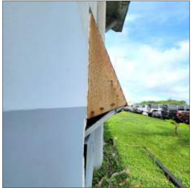
Figure 2: Exhaust Vent to be Removed and Replaced
