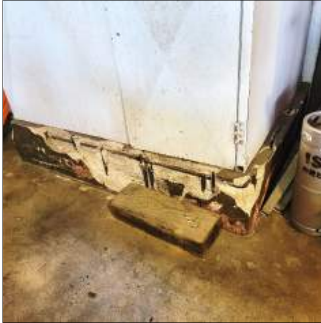
Figure 19: Bathroom Foundation to be Repaired
