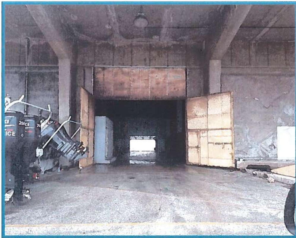
Bay 2 Landside: PAG CIP/Safety Roll-up Door 20'x20'
